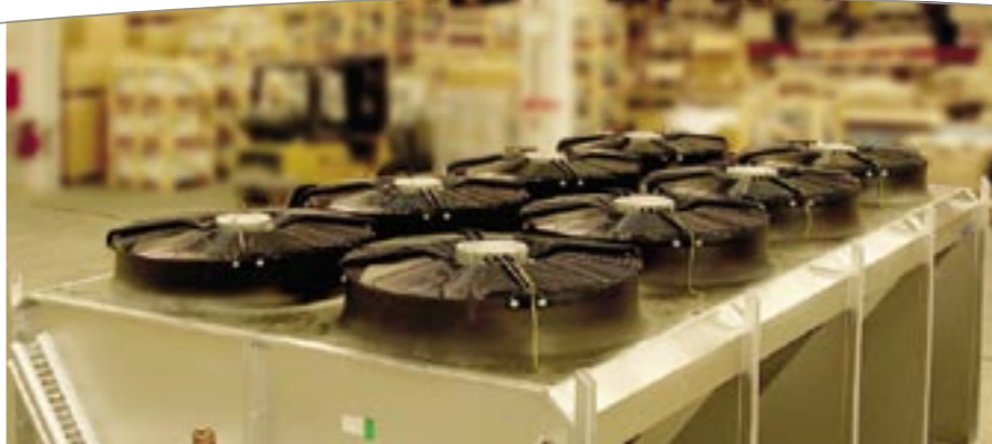
Meticulous control of fans saves energy and keeps noise and draft at a minimum.
